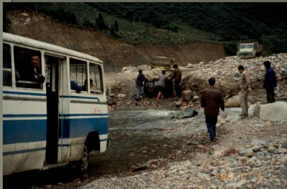
Washed out road
